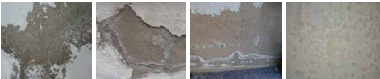
SAMPLE PHOTOS OF UNSUITABLE SURFACE WALLS
